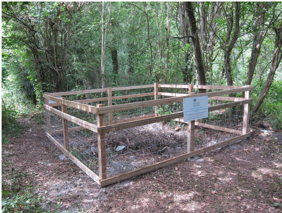
Figure 14, Partially collapsed shaft recently fenced by Coal Authority Marked 'Old Shaft on 1927 OS map. SJ 6809 0195. S Dewhirst 2018
