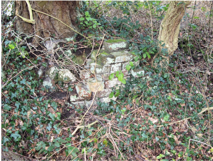
Figure 15 Brickwork in rectangular depression – probably the site of the Winding Engine/Boiler. SJ 6809 0192.
