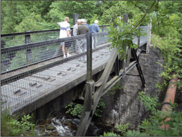
Pontycafnau, the 1793 cast iron tramroad bridge from the Gurnos limestone quarry which also carried two water feeders to the works
