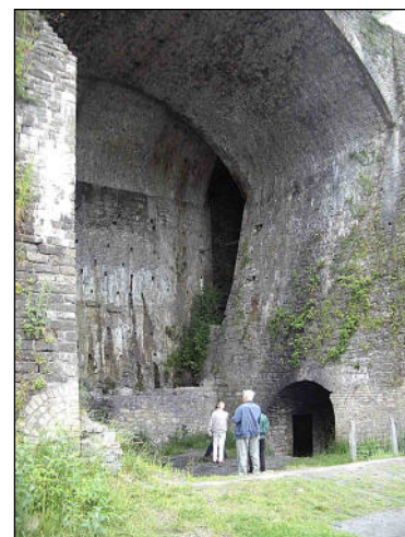
One of the huge furnaces of the Cyfarthfa Ironworks which were the source of the Crawshay empire and the main rivals of the Guests in trade
