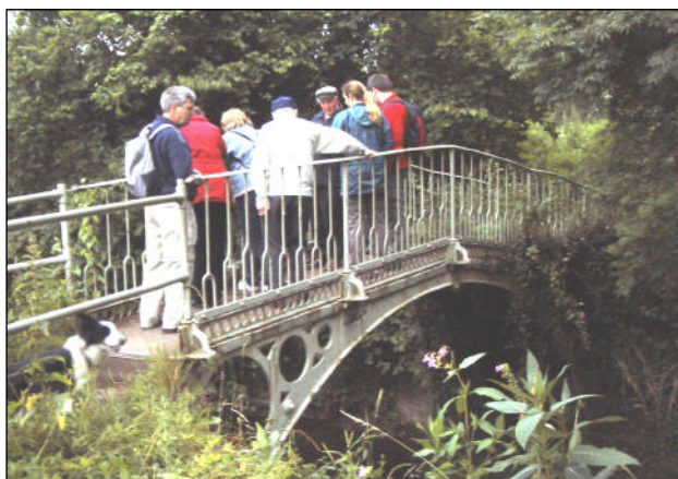
This iron bridge over the Stour is a smaller version of its more famous namesake
