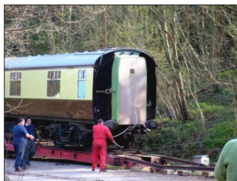
Rolling the carriage off the trailer and on to a temporary stretch of track
